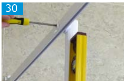
Ensuring the post is straight, pilot drill through both the curtain rail and post using a 3.0mm drill. Screw both together with a No8 x 38mm pan head screw and cap.
