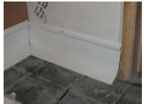
Ensure the coving fits neatly at both the corner and architrave points
