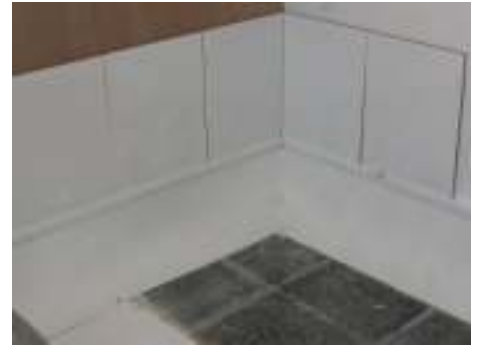
You can now tile your walls. Use silicone sealant to form a seal between Contour coving and the tiles
