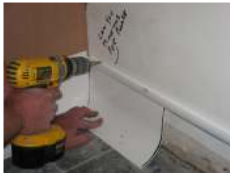
Fix the modified Contour coving in position. Ensure that it fits neatly at the corner and architrave
