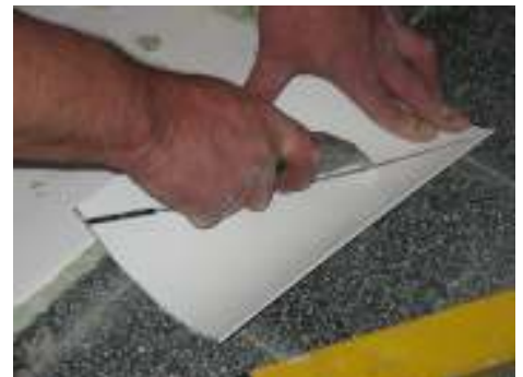
Take the cut-out section, cut diagonally from the bottom edge of the coving cut-out to approximately 20mm below the top corner
