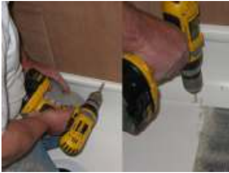
Screw the coving to the wall through the tiling lip. Pilot drill and screw to the floor former
