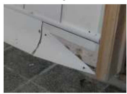
Secure the bottom edge of your cut-out to floor. You should now have a tapered profile finishing at the door
