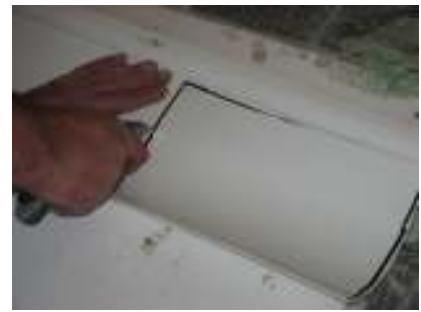
Measure back approximately 300mm from the architrave towards the corner and mark and cut out a rectangle
